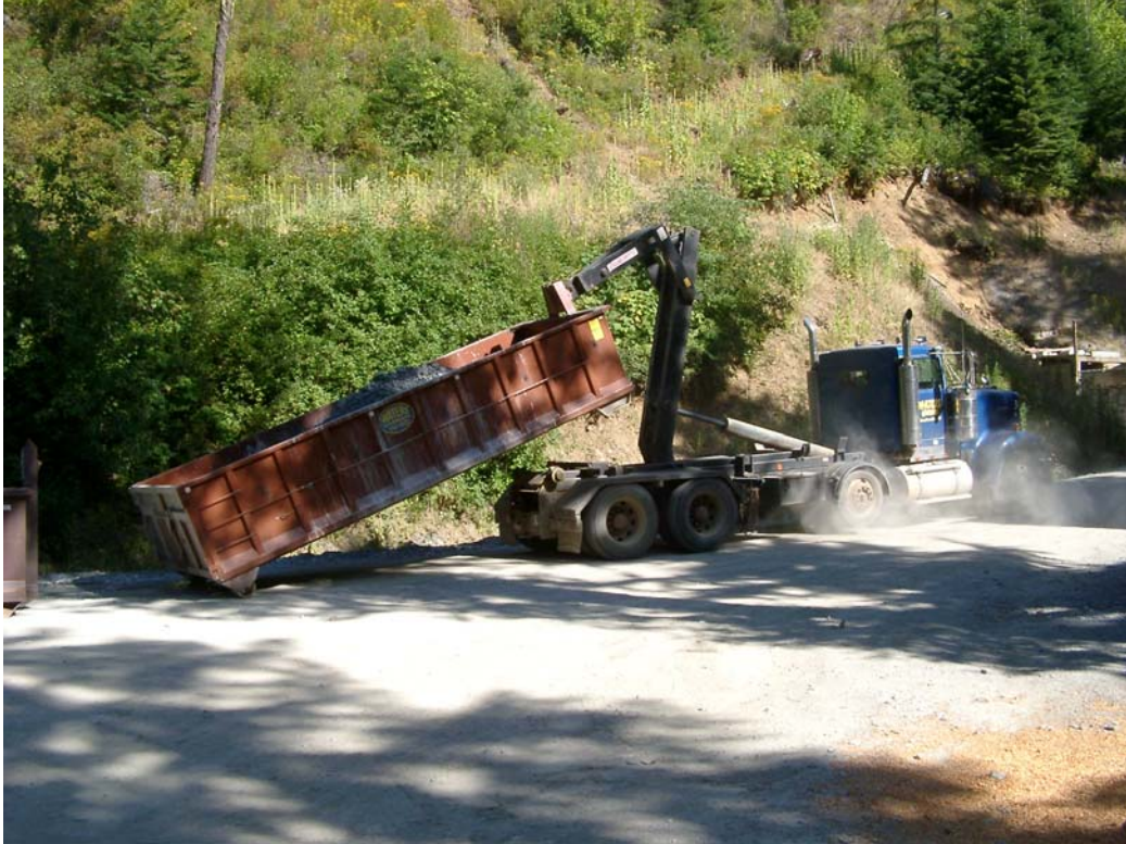
Figure 3: New Jersey Mining Company's Golden Chest mine. Uploading the ore bin for transport to mill; mine portal is on far right.
