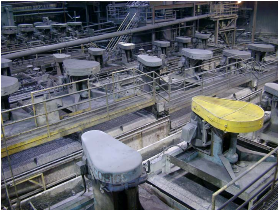
Figure 4: Thompson Creek mine's flotation cells in mill.
