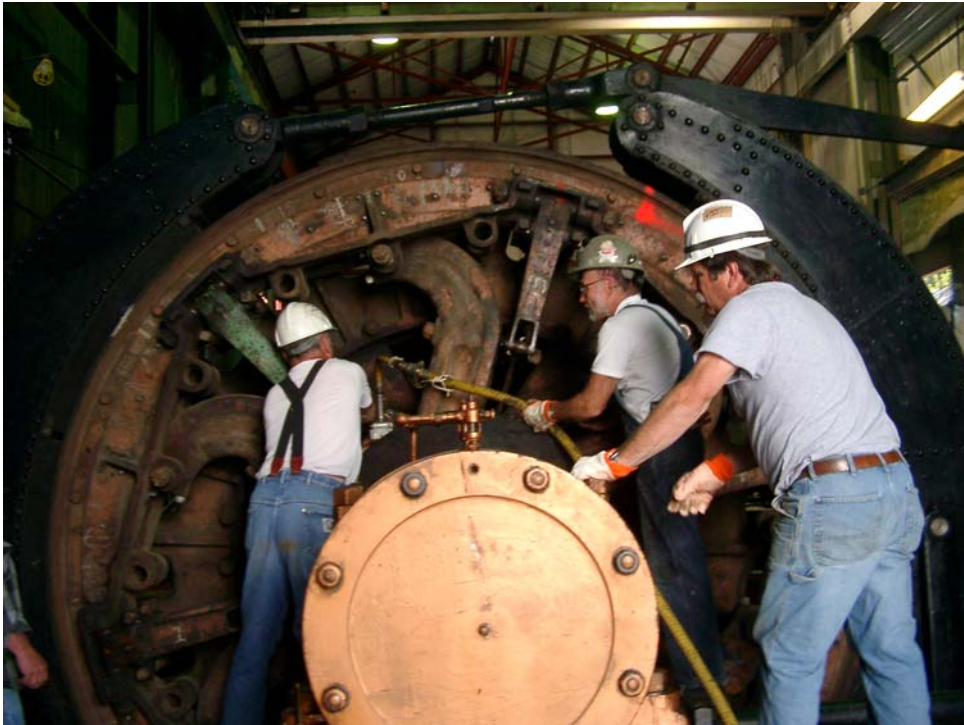
Figure 2: Sterling's Sunshine Mine. Workers are detaching the old cable from drum before installing new cable for the Jewell Shaft hoist.
